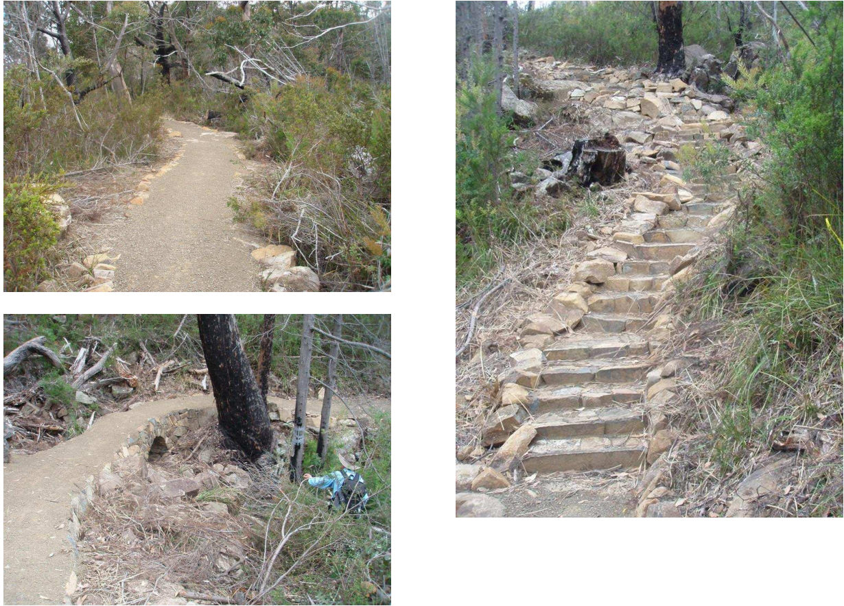
Figure 1. Recent photos taken of the Cape Haury track which is under construction (Source, HWC).
